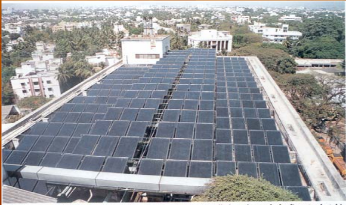
IREDA financed 42000 LPD Solar Water Heating System installed on the roof of a five star hotel in
